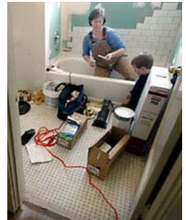
Nashville resident Elizabeth Stelling installs tiles on the wall of a bathroom at the home of a client off Gallatin Pike. It's work Stelling says she does on contract since losing a teaching job at Harpeth Hall School because of an ordeal with identity theft. JAE S. LEE / STAFF
